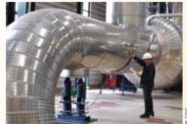
The Bugey NPP turbine hall
